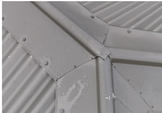
Ensure sealed- All areas to comply
